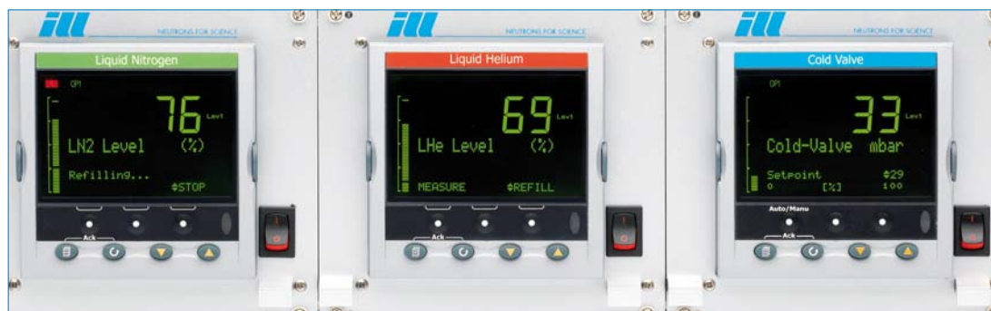
Figure 8: Cryogenic control systems showing the cryogenic fluid values and cold valve pressure.
