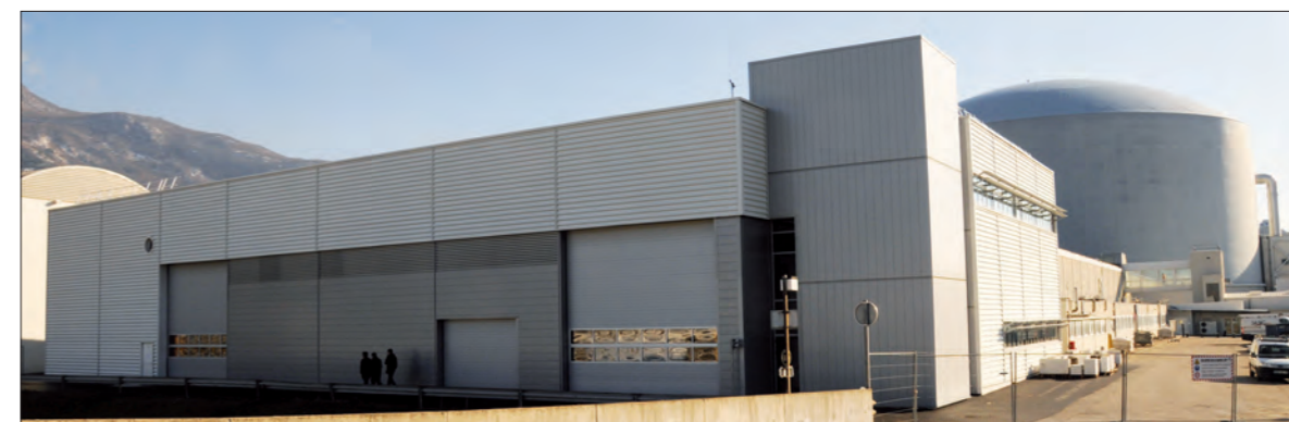
The extension of the ILL7 guide hall - which is now 118m long - was completed on 8 November, right on schedule.
