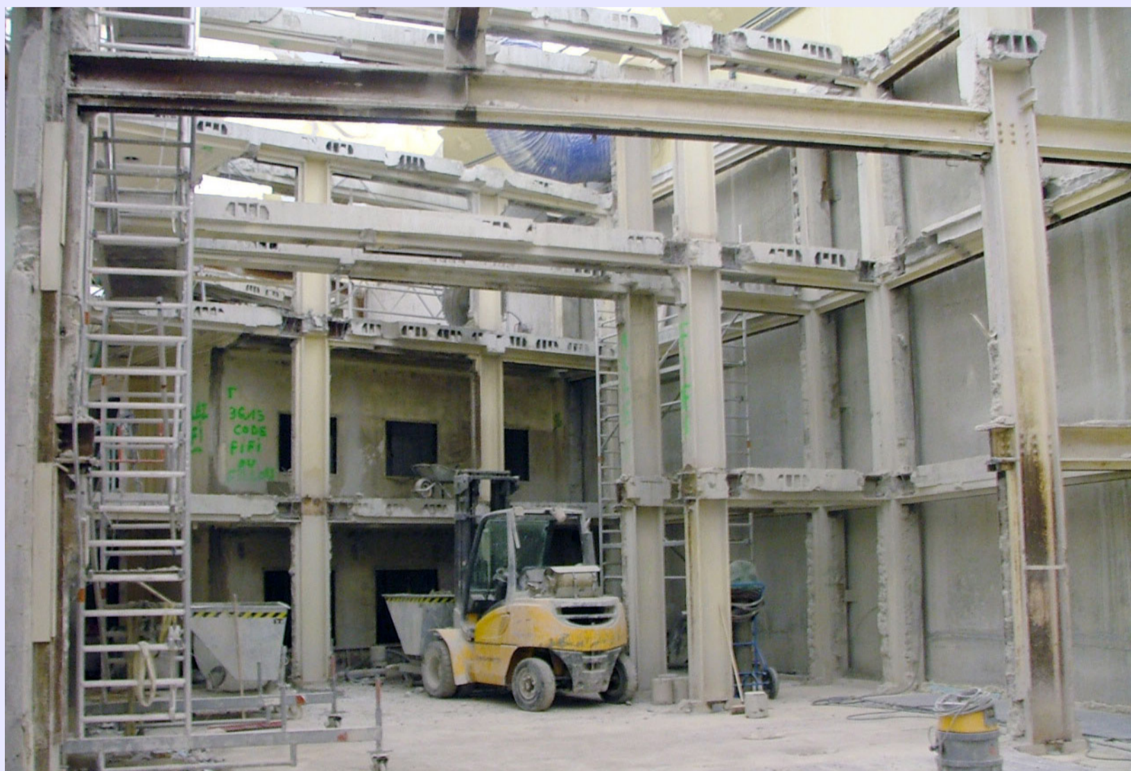
Fig. 11.6: Demolition and removal of internal structures at the top level of the ILL building to reduce inertia in case of a seismic event.
