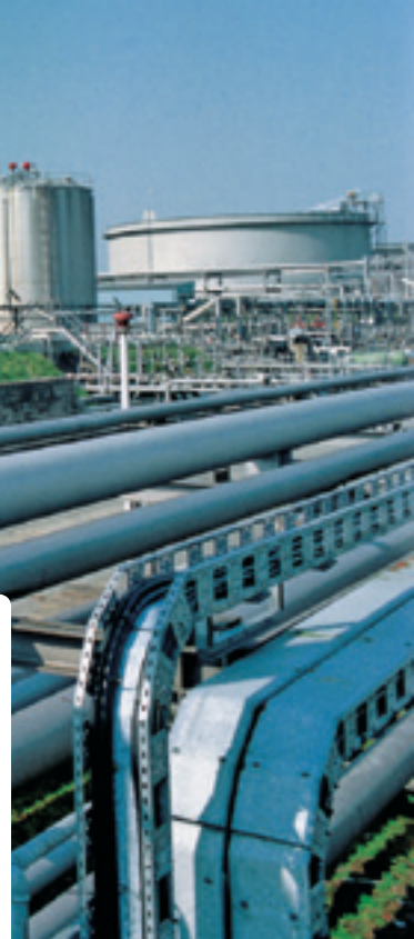
Siemens is investigating the thermoelectric generation of electricity using waste heat from industry
