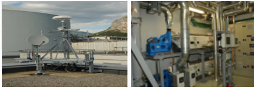
FIG.6. Communication tools and air conditioning systems of PCS3
