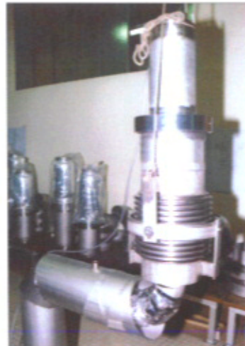
Cryogenic line for ARIANE V vacuum chamber
