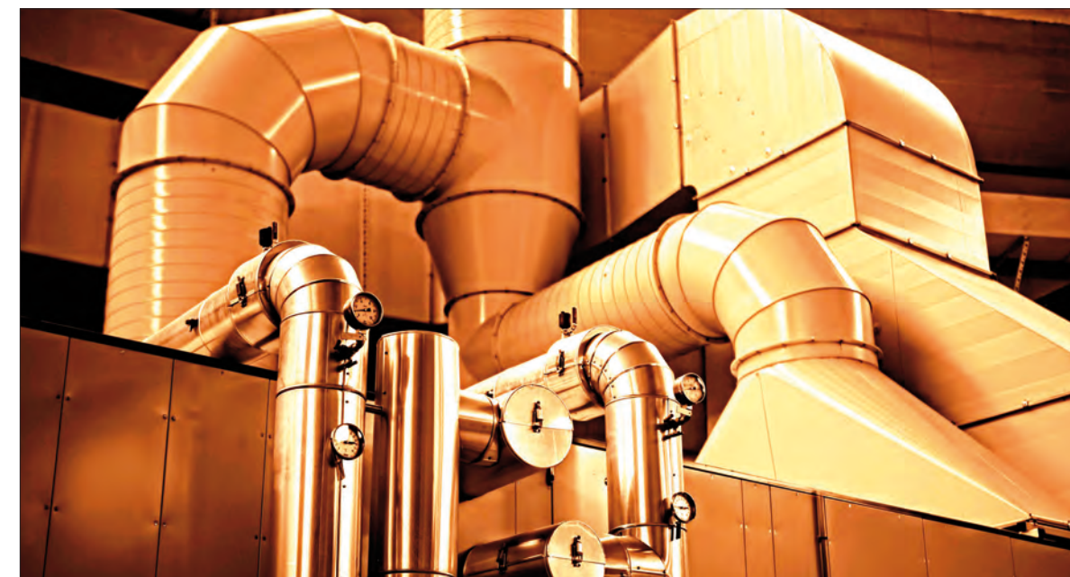
The new air-conditioning system for the ILL reactor. Copyright: Bernhard Lehn, Fotodesign, studio@bernhardlehn.de.
