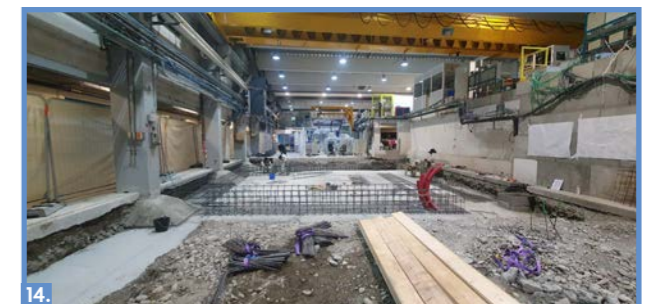
11. Ground preparations for the new H24 instruments. 12. Guide pass-thoughts from the reactor building to ILL7. (Ch. Monon) 13. Installation of the new twin neutrons guides of H24 . (P. Lachaume, Ch. Monon) 14. Preparation of the new D10+ zone.
